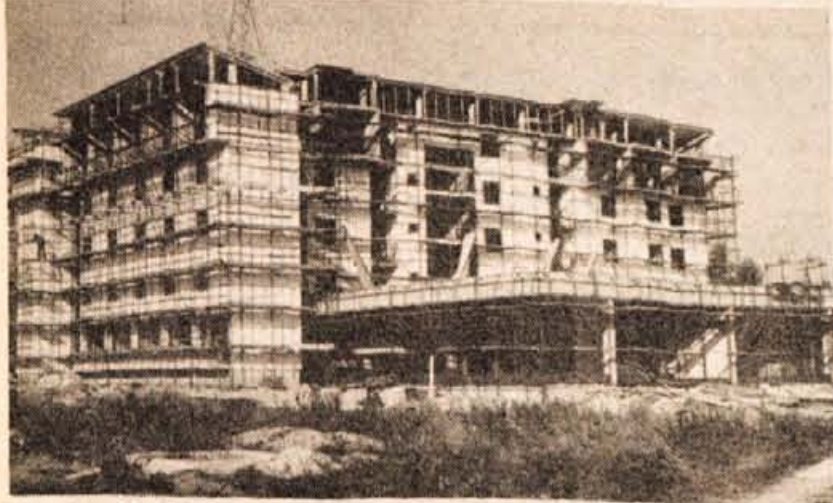
Kranj - Na Zlatem polju je spomladi začeta gradnja Dijaškega doma... (Text continues describing the construction project in Kranj, mentioning the future of the building and the local school.)
